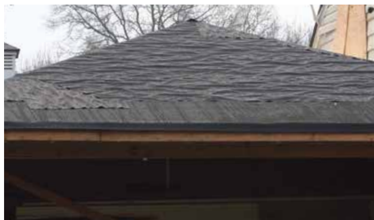
Conventional organic felts can absorb moisture, causing severe buckling and wrinkling—and a terrible-looking roof
